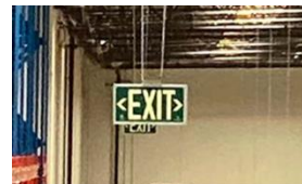
Exit Sign hung from ceiling
